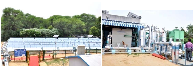
Fig. 3: 100kw solar cooling system at SEC, Gurgaon
